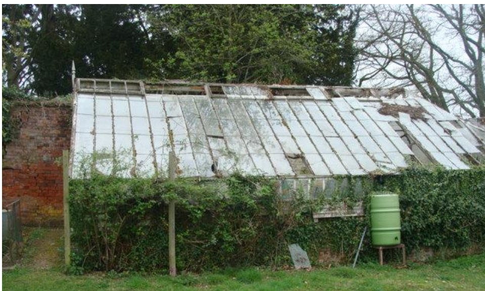
Picture 30. Greenhouse within walled garden to north of Garden House. In deteriorating condition but still capable of repair.
